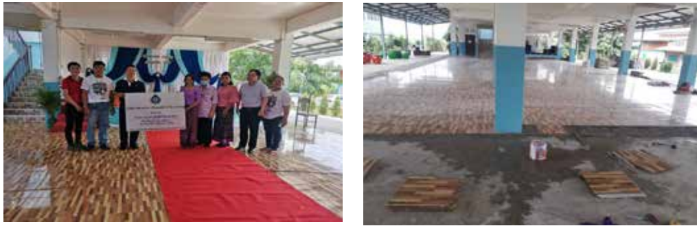
On September 26, 2020, Thai Agro Energy Plc. handover the project of tile basement floor of Baan Mai kilo 8 School. Dan-chang district, Suphanburi
